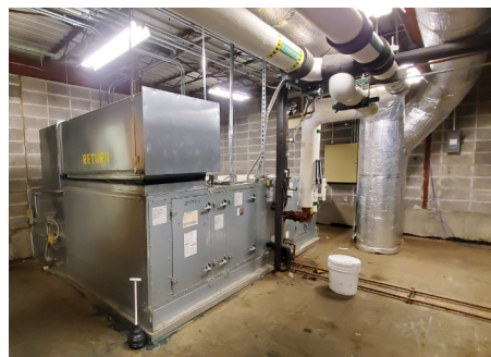
Air Handling Unit at Kansas City Kansas Public Library 1
