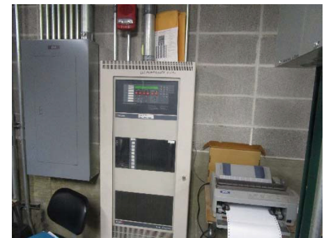
Main Fire Alarm Panel in KCKPL 2
