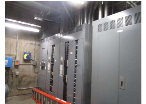
Main Electrical Switchboard in KCKPL 1
