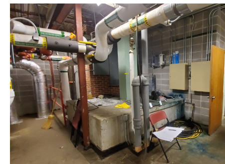
Mechanical Room at Kansas City Kansas Public Library 1
